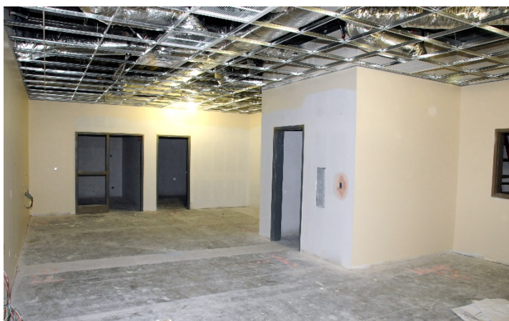
Figure 2. Proposed section of the 6500 Building dedicated to and prior to construction of the BPL.
